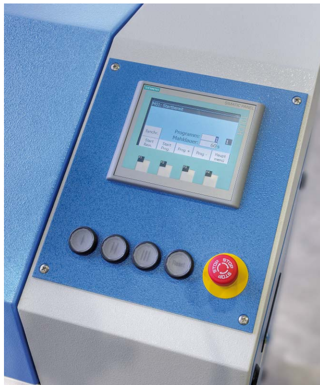
Touch screen operating panel
